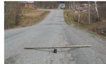
Lesson 1 Permanent Deformation
